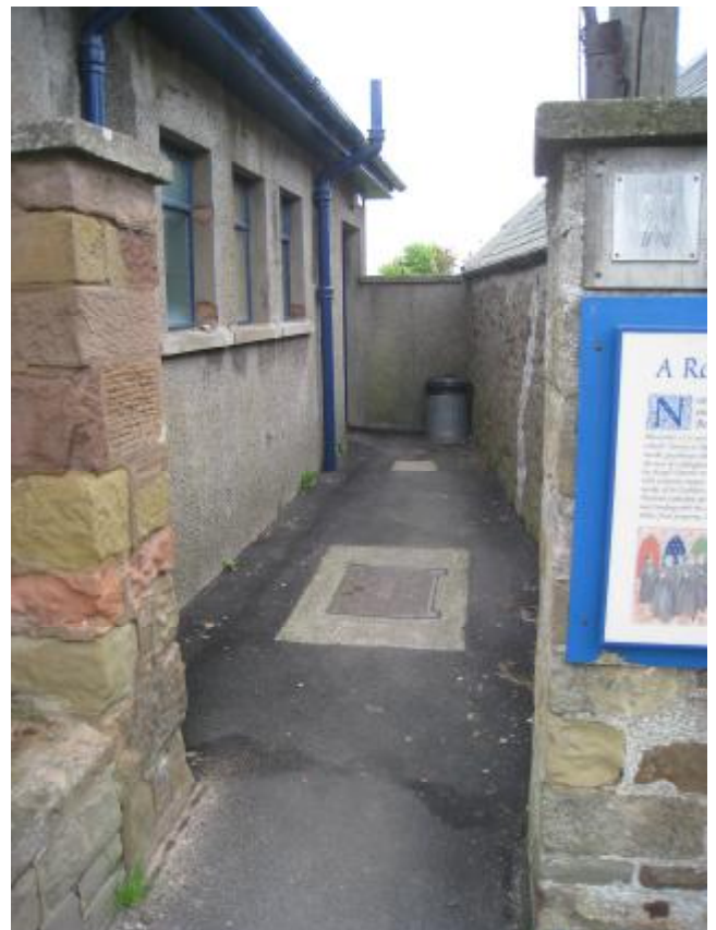
The existing gap between the toilet building on the left and the old mortuary building on the right.
